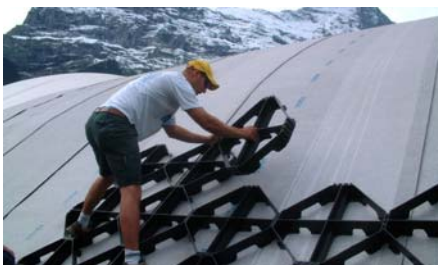
The Georaster® elements are installed from the bottom up. In the background, the legendary Eiger North Face.
