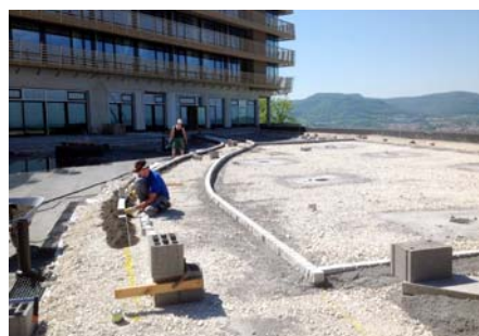
Gravel is being applied above the Floradrain® FD 40-elements to provide a base for the natural stone paving.
