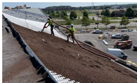
The substrate is blown on roof. Floraset® FS 75 elements were chosen for slopes up to 25 degrees.
