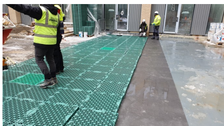
The heavy duty RXS spacers were laid on all podiums allowing them to be used as roof gardens with hard and soft landscaping.
