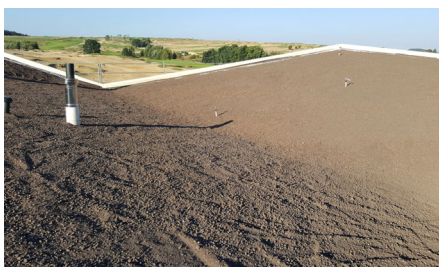
The roof area after application of the System Substrate "Rockery Type Plants".
