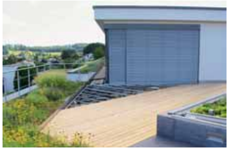
This surface rises from the threshold towards the perimeter to get sufficient space for a green roof application.
