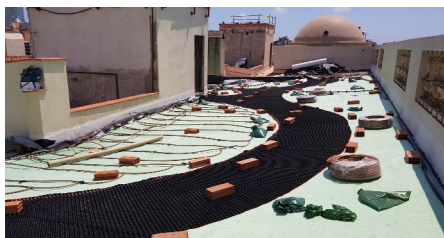
The drainage and water storage elements Floradrain® FD 40-E are installed across the entire roof and Aquafleece® AF 300, with its driplines, is installed in the plant areas for underfloor irrigation.
