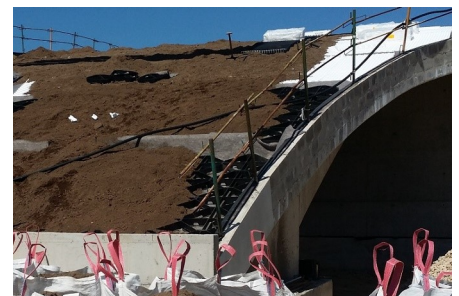
Floraset ® FS 75 and Georaster ® elements were installed in the the pitched and steep pitched
