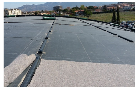
Stable shear barriers were concreted onto the roof and sealed in order to transfer the shear forces into the roof structure. The Protection Mat BSM 64 was laid on top of the root resistant waterproofing
