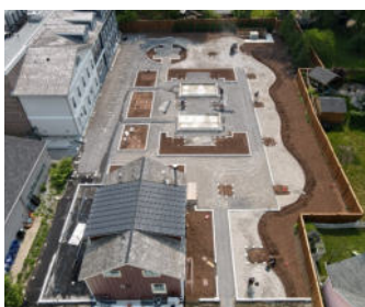
The roof area under construction shortly before laying the terrace slabs and planting.
