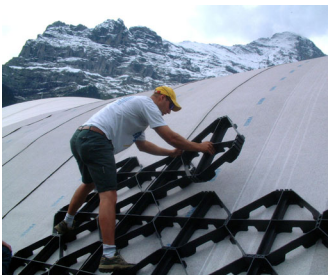
The Georaster® elements are installed from the bottom up. In the background, the legendary Eiger North Face.
