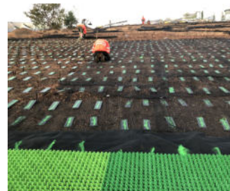
The substrate underneath the plastic mats lies embedded between two layers of geogrids.
