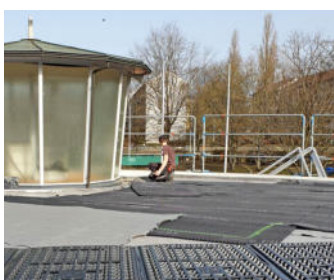
The drainage and water storage element Floradrain® FD 25-E was laid fully surfaced. Additional Solar Base Plates SB 200 were placed in the areas under the solar system. © Hohenschläger/Zinco
