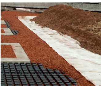
Floradrain® FD 60 elements were applied and infilled with Zincolit® Plus on this entire roof surface, also in the plant troughs which were meant for olive trees.
