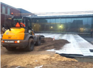
This photo shows the sequence of all layers from the waterproofing to the base layer.
