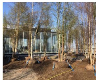
The root balls are anchored to the ground to withstand the high wind loads on the roof.
