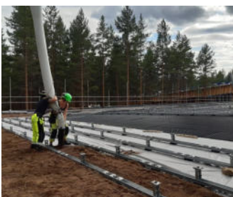
To make use of the seeds in the retained forest soil, it was combined with the green roof substrate.
