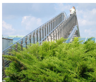
After more than 8 years the vegetation on the roof is still in excellent condition.
