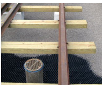
Installation of the green roof build-up under the rails. The drainage layer consists of infilled Floradrain® elements.
